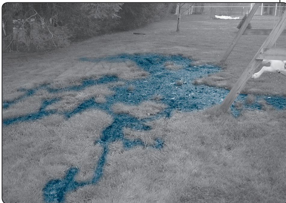
Damaged, waterlogged areas in the lawn over the drainfield indicate drainfield system failure.
