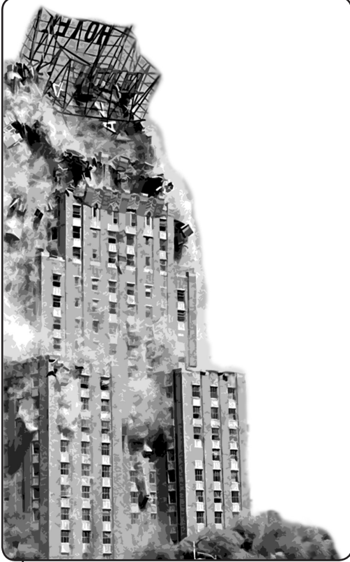
Controlled demolition of abandoned buildings creates tons of rubble. If graded and sized properly, this waste material can be used as a substitute for native gravel in drainfields.
