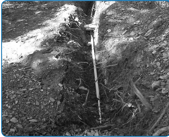
This photo shows a water line crossing under a sewer line. This arrangement violates health codes in every state because a sewer leak could contaminate the water line below. (Photo by Allen Marchan)
