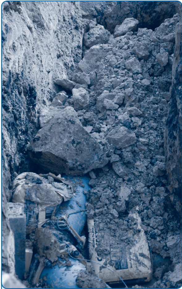
The backfill seen in this photo is of a much larger size than recommended. (Photo by Julie Black)
