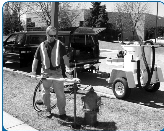
When a water main breaks in the middle of a frigid night, you'll be glad the valves function correctly.
